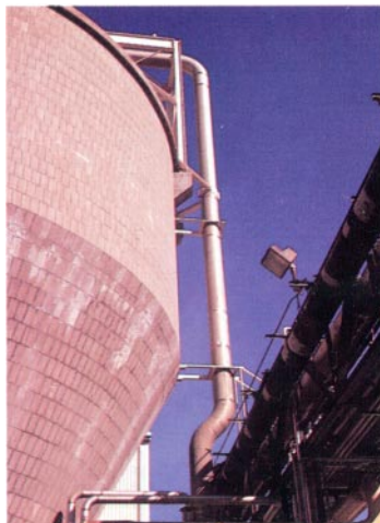
24" diameter stainless steel pipe used in the pulp and paper industry to load pulp into a bleached pulp stock chest.
