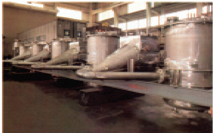
Stainless steel nitration system.
